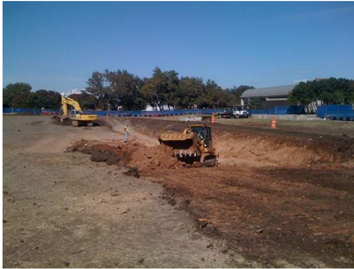
Excavation site of the Kimbell Art Museum's expansion--a building designed by Renzo Piano. Clay collected here was used in the creation of Adam Silverman's Reverse Archeology project (2010 - 2012), an installation of three pots produced expressly for the Museum's 40th Anniversary. Photo credit: Adam Silverman
