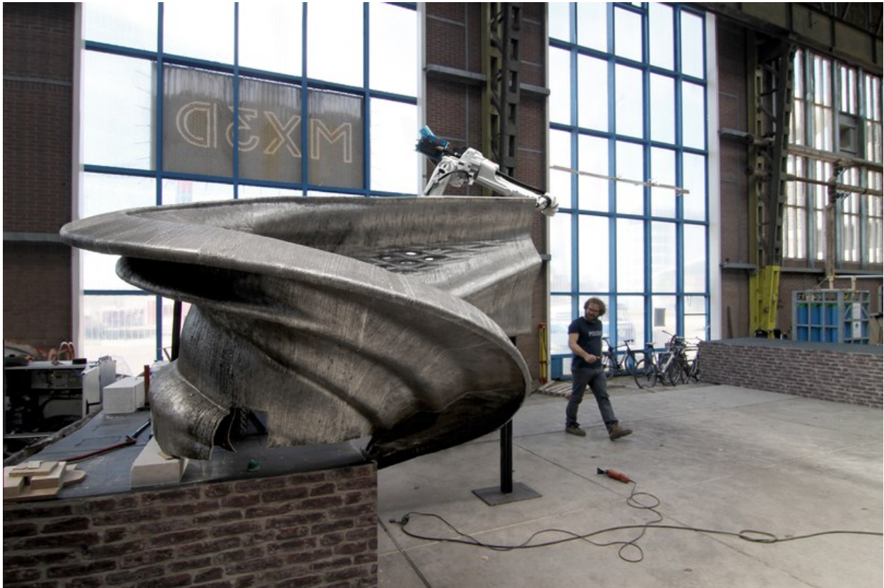
A closer look at the bridge, which will feature a swirling end that anchors itself to the canal wall.
