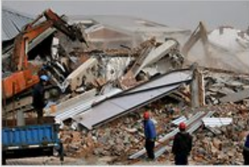
On Tuesday, workers were demolishing the Shanghai studio of the Chinese artist Ai Weiwei.
